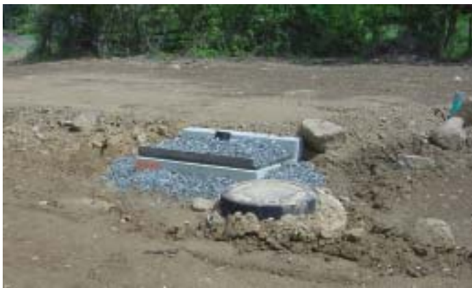
An example of improper installation. Overflow pipe is not adequate.
